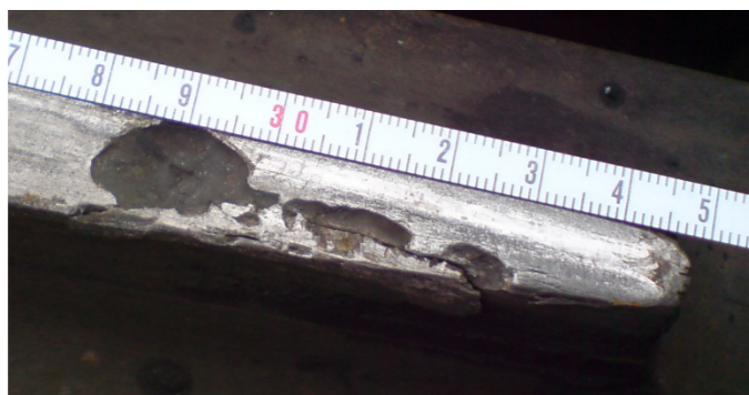
Figure 4 – Breaking of the core of the VAE cross 60E1 1/11 and cracks at the Alotene station
