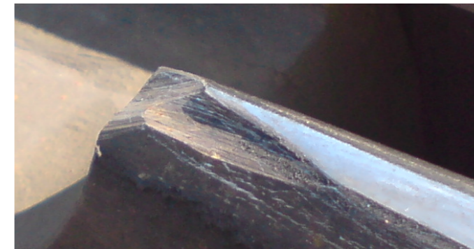
Figure 6 – Breakage of the end of the core of VAE cross R-65 1/9 at the Skirotavas station
