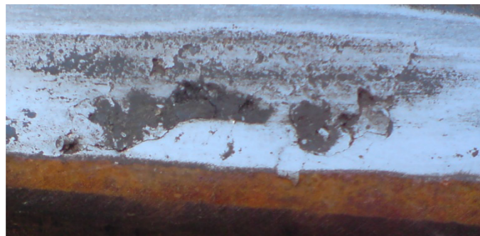
Figure 8 – VAE cross 60E1 1/11 cracks at Slampes station
