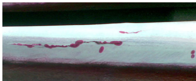
Figure 15 – VAE cross 60E1 1/11 core longitudinal crack at Crust station
