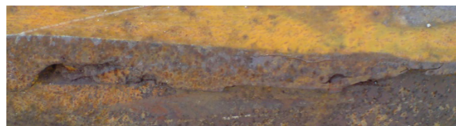
Figure 9 – VAE cross-cross R-65 1/11 detachment at Slampes station
