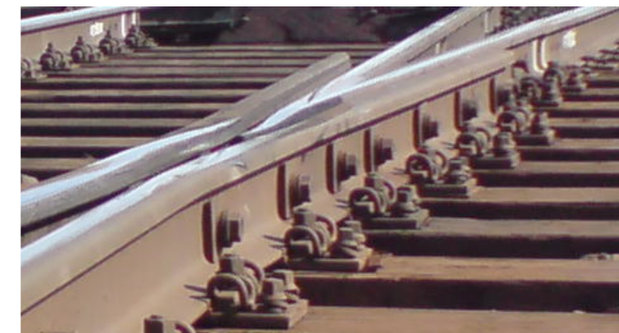
Figure 7 – VAE cross R-65 1/11 worn core at the Aizkraukle station
